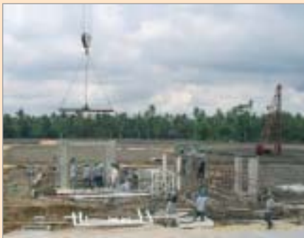
Progress in the construction work on the "24 Day House". This is the situation on the third day
